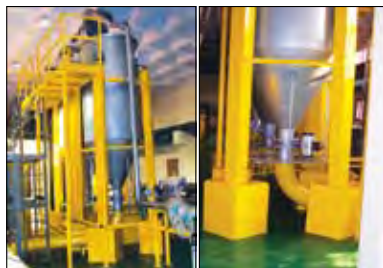
Fig. 5.29 (a) Piping, Weighing Tanks and Support Structures (b) Weighing Tank, Drain Valve and Platform for Calibration of Tank
